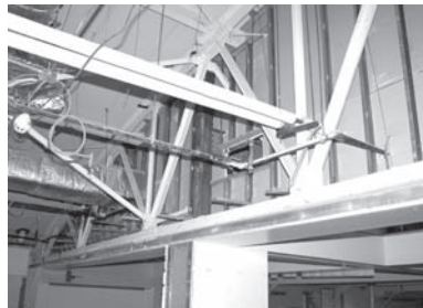
The curved roof of the old boy's gymnasium can be seen as the walls and ceiling are removed.
