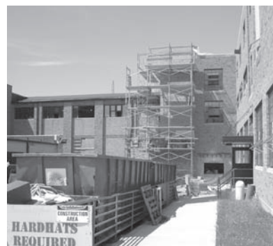
The elevator being constructed on the south side of the school is part of the new accessibility plan.
